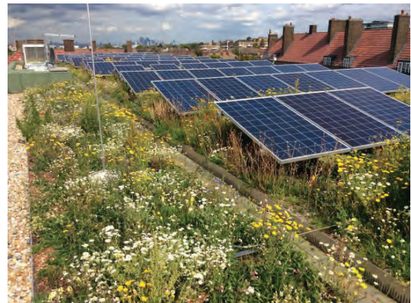
Example of solar photovoltaic panels being incorporated with greenroof elements (guideline 94 and 95).
